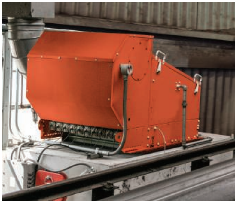
FIGURE 6. Integrated air cleaners are smaller, independently operating units at each dust-generation point
