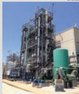
FIGURE 7. The divided wall column at the University of Texas at Austin's Pilot Plant is controlled using WirelessHART networking technology
